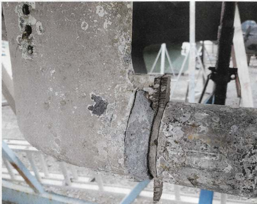
The protective coating on this saildrive is failing and needs to be renewed after a thorough cleaning. Corrosion is beginning to take hold and both anodes need to be replaced
