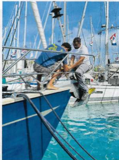
6. Aqualuna lost her forestay; (right) riggers get to work repairing the forestay on Aqualuna
