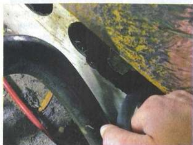
This black cable for the wiring loom was rattling loose
