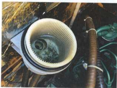
Weed in the seawater strainer
