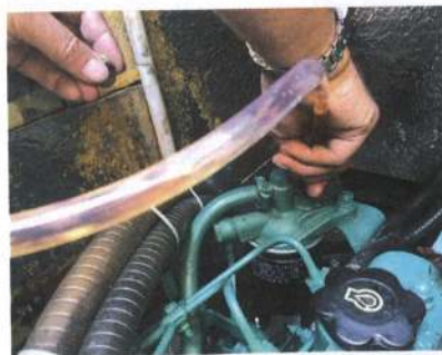
Clean fuel drawn into the secondary filter using the oil change suction pump. Note bleed plug in Stu's left hand
