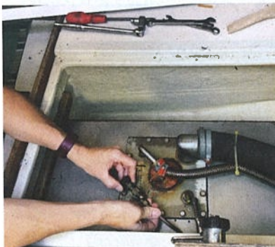
Undoing fuel lines ready to remove the inspection hatch of the fuel tank
