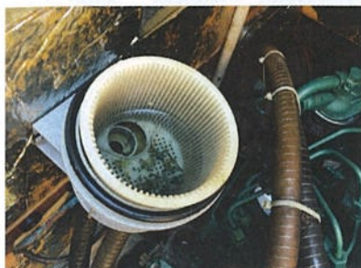
Weed in the seawater strainer
