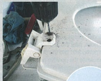
Rusted hinge screws had to be drilled out.. leaving oversize holes which Stu filled with epoxy before replacing with new stainless steel screws
