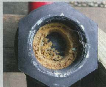
An example of limescale build-up
