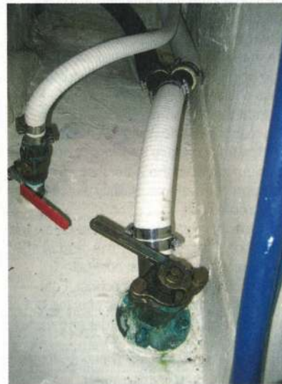
The waste pipe seacock is closed to trap in the descaler
