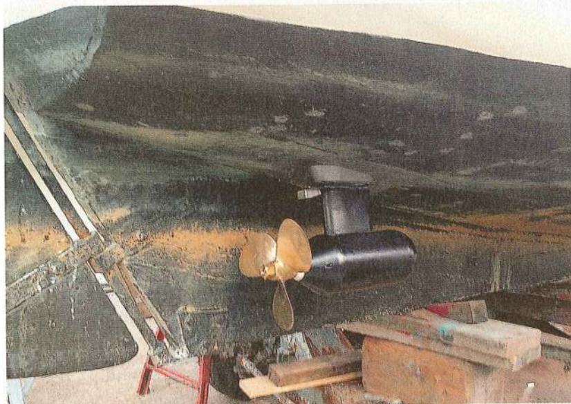
The saildrive bolts through the planking, with the cables being led up into the boat
