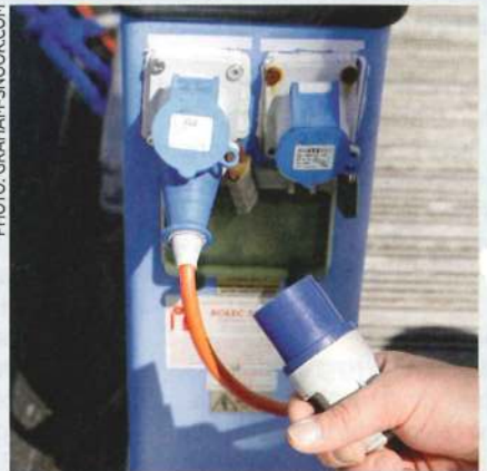
Consider unplugging the shore power for the first night, while you're still alongside. Can the batteries cope with the load?
