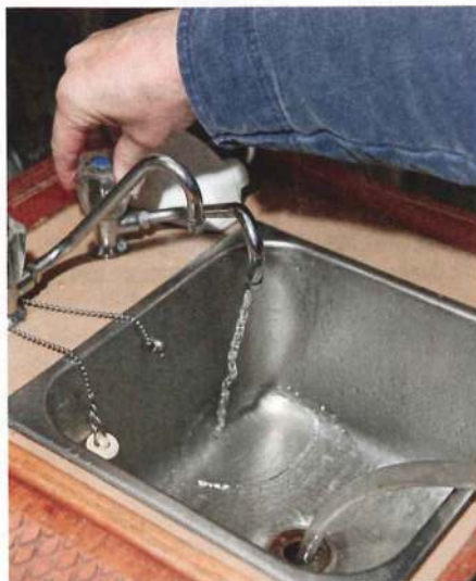
Drain water tanks and leave taps open
