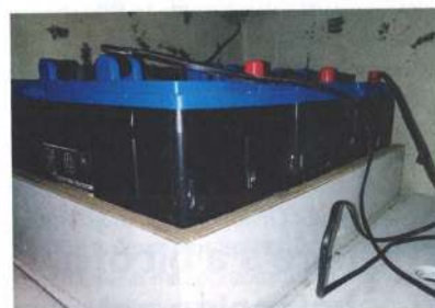
The three new Exide batteries wouldn't fit in the engine room but we found space for them to the aft of the boat under the cockpit. A box fixed to the boat keeps them secure
