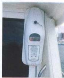
An easily accessible EPIRB behind its cover
