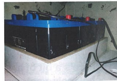
The three new Exide batteries wouldn't fit in the engine room but we found space for them to the aft of the boat under the cockpit. A box fixed to the boat keeps them secure
