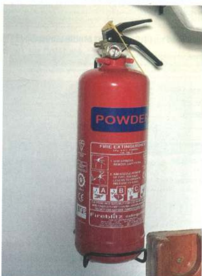
At least two fire extinguishers are essential
