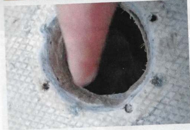
LEFT When changing deck fittings on a balsa core deck, preferably an internal plywood patch should be glassed in
