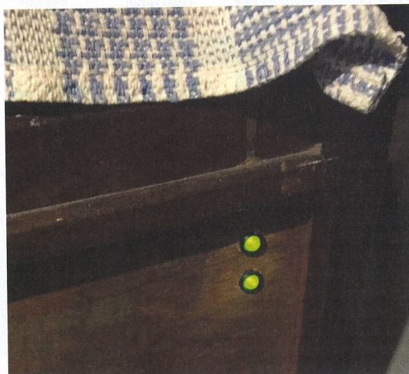
The battery monitor LEDs installed under the bunk
