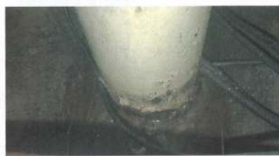
What about the base of the mast support post? This is a critical structural part of the boat, yet is often neglected
