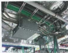
An HVAC distribution hub set into the deckhead of a superyacht. The entire network can be centrally controlled by the skipper, cooling only those areas that are in use
